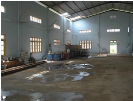
Workshop with roof damages
