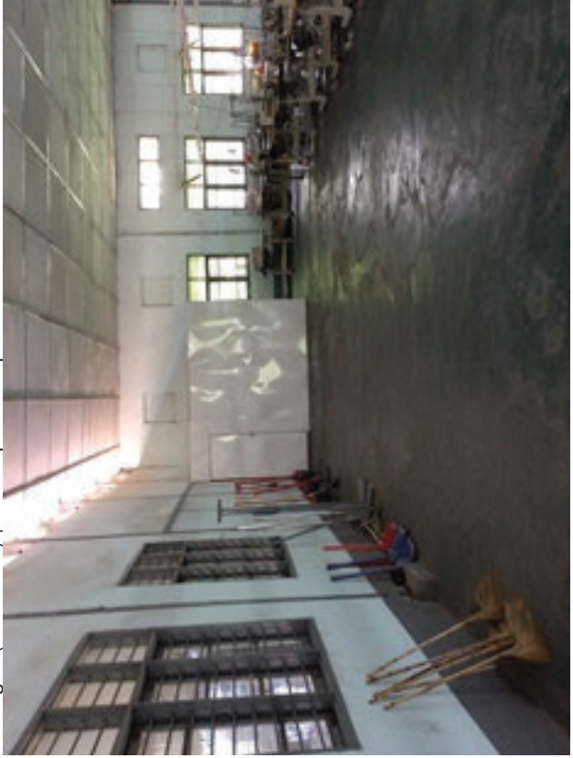
Leakages (roof / floor) | Room part with provisional store room
