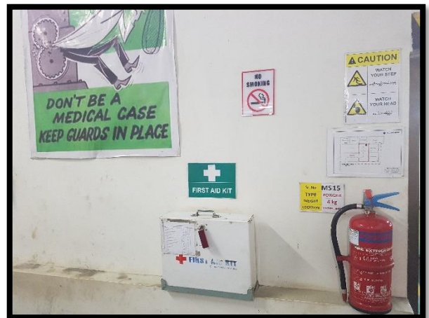
Firefighting and First Aid equipment available
