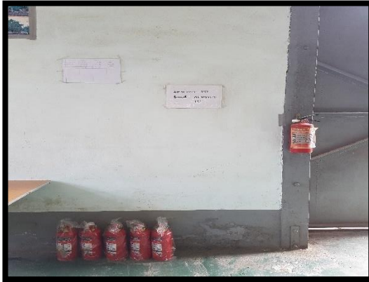
Firefighting equipment is enough
