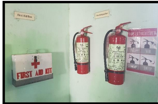
Firefighting equipment available
